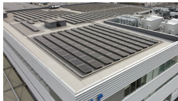
Solar power generation at the NP Building of the Fujisawa Plant
